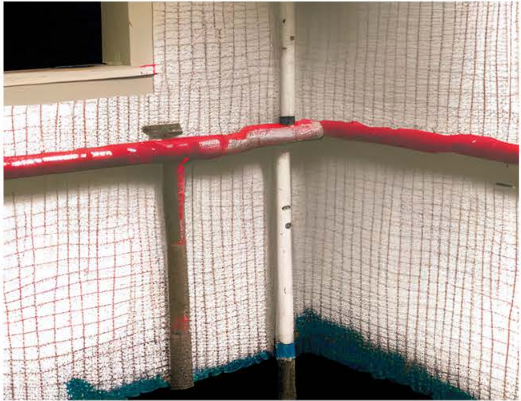
Hysteric pipes and wall
