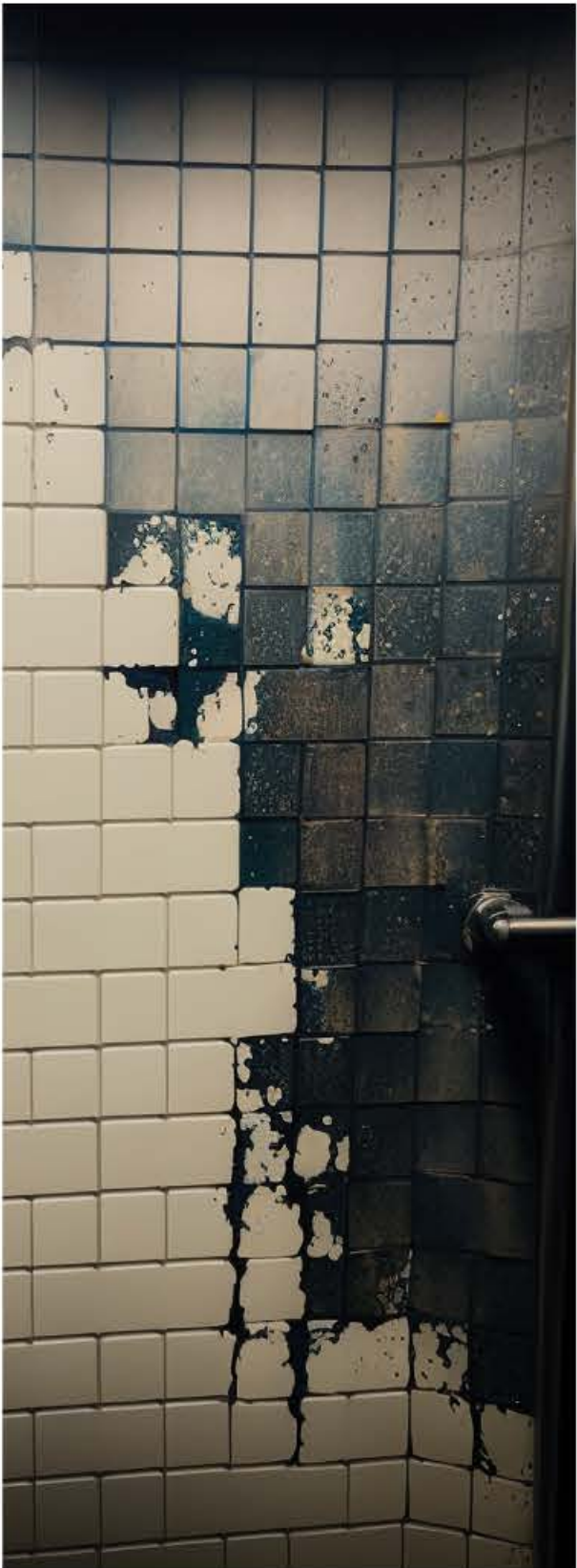
A depressed bathroom tile
